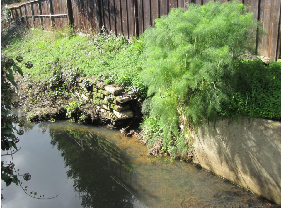
View of erosion on bank of West Creek from Cecilia Way Bridge looking south/downstream.
